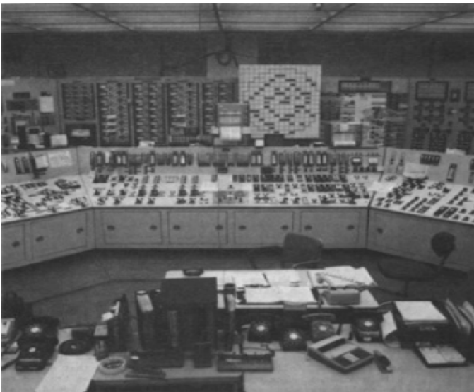
Figure 1. Three Miles Island control room (Kenemy, 1979, p.112).
